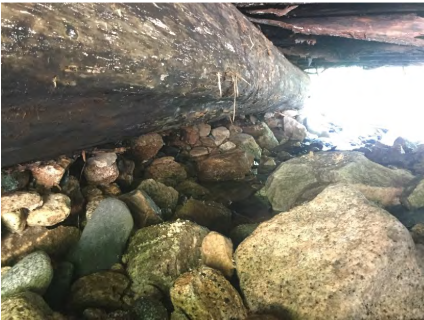
Left Abutment Scour
