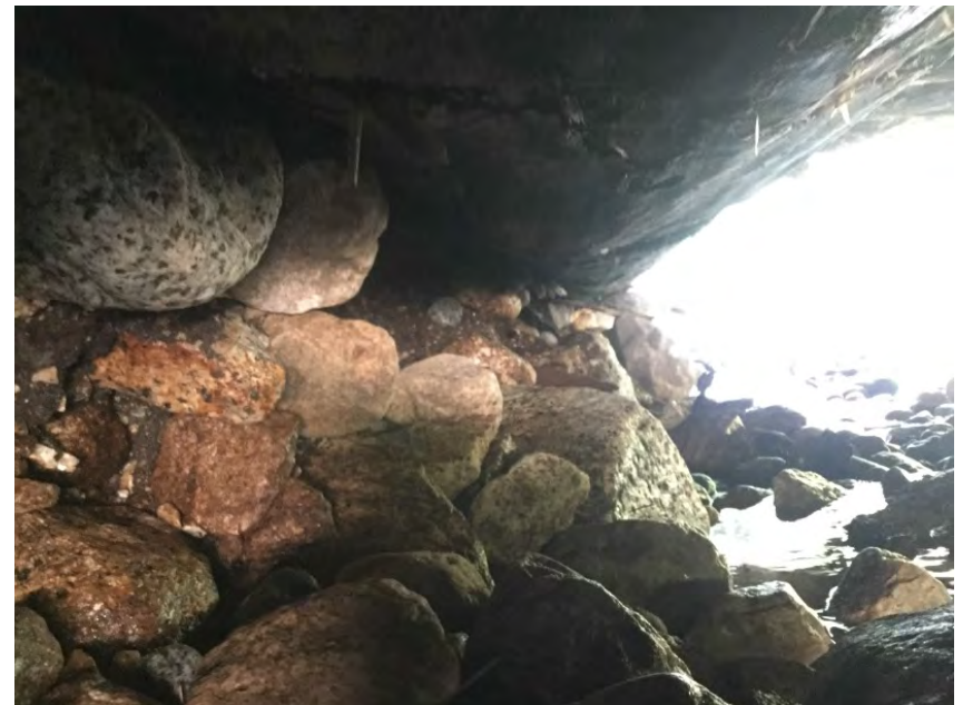
Left Abutment Scour
